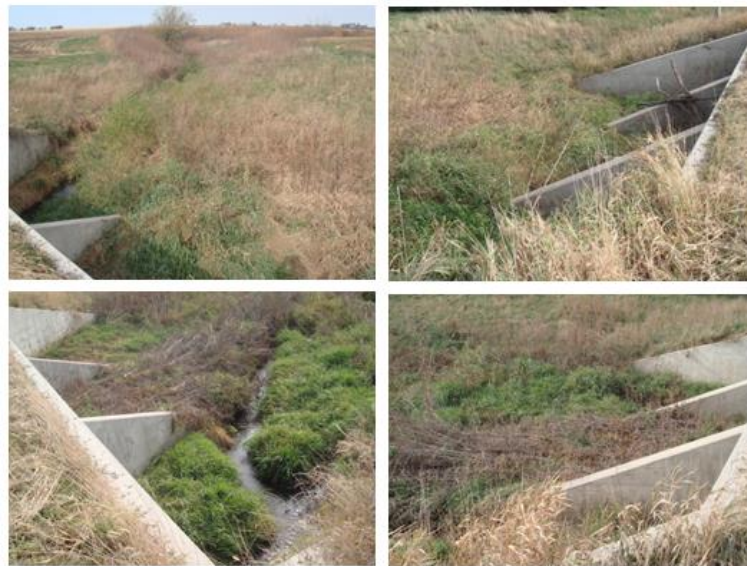
Figure 1.11 Culvert siltation observed through previous studies (M Muste et al., 2009): a) 3-box culvert located on the Old Mill Creek in Solon; b) 3-box culvert located on the North Branch Volga River
