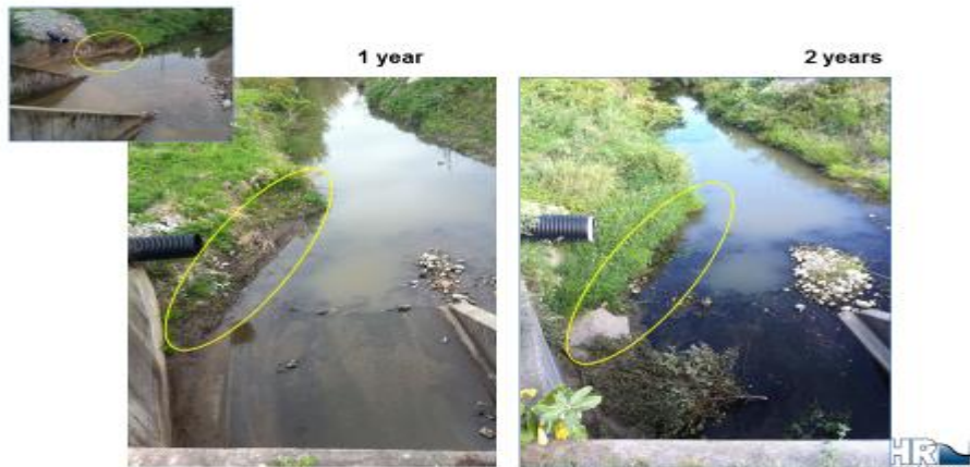
Right culvert box: deposition evolution after cleanup
